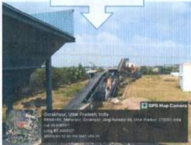
C & D Waste Processing Facility
